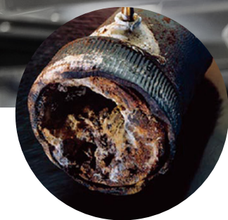
Picture of a blockage in a sewer
